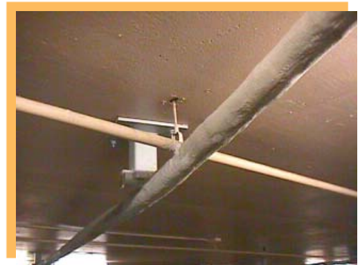
Fireproofing on grounded external tendons
