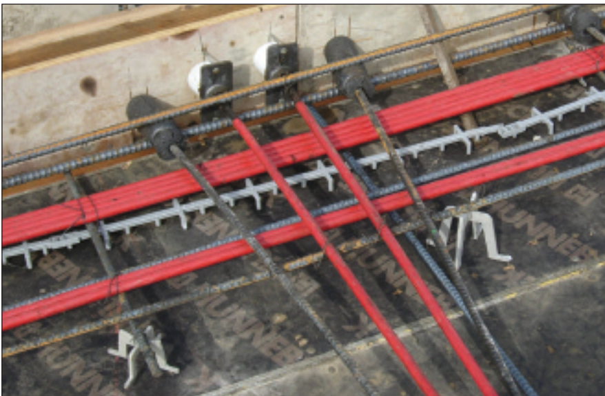
Top: To prevent restraint, plastic is placed along the top of a wall that the slab is crossing. Bottom: The black foam rubber around the first few inches of the dowels coming out of the adjacent wall will allow the post-tensioned slab to shorten during tensioning without cracking the slab.
