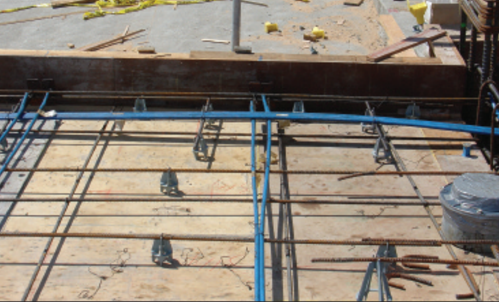
These tendons will create a downward force that is nowhere near a band or a vertical support and that can cause cracking or a small blowout.
