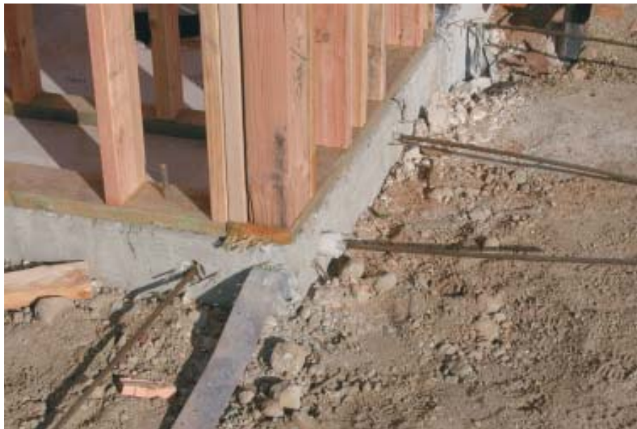
Figure 5. Tension-end fittings are first nailed to the forms (top) before the tendons are threaded through a hole in the perimeter form. The hollow plastic pocket former will be pulled out when the forms are stripped, leaving a recess for the nosepiece of the hydraulic ram used to tension the tendons (above).
