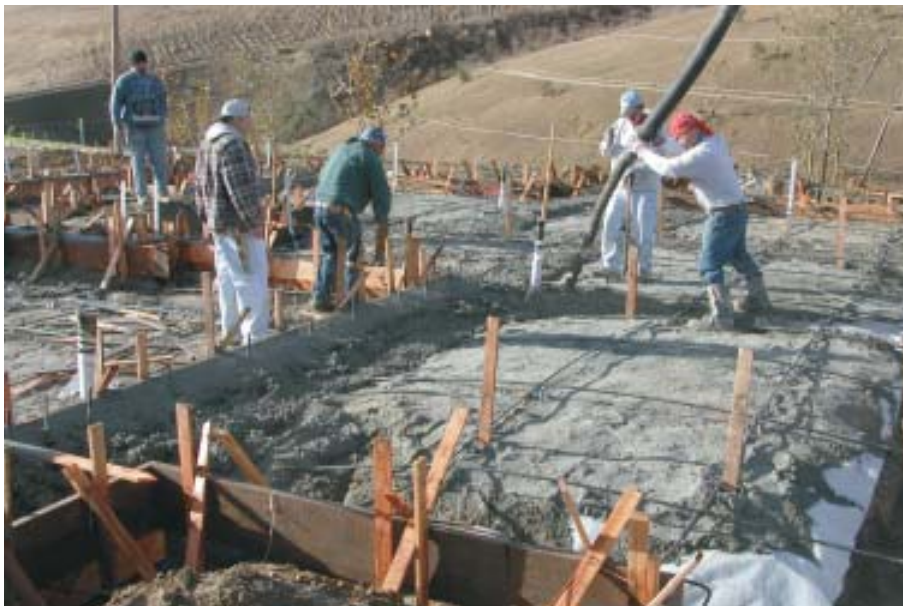
Figure 7. The concrete crew will finish filling the perimeter footings and internal ribs before pouring the slab. The wide spaces between tendons make it easy to walk around on the subgrade without tripping over the reinforcing — something that's much harder to do on conventional slab reinforced with wire mesh or a closely spaced rebar grid.
