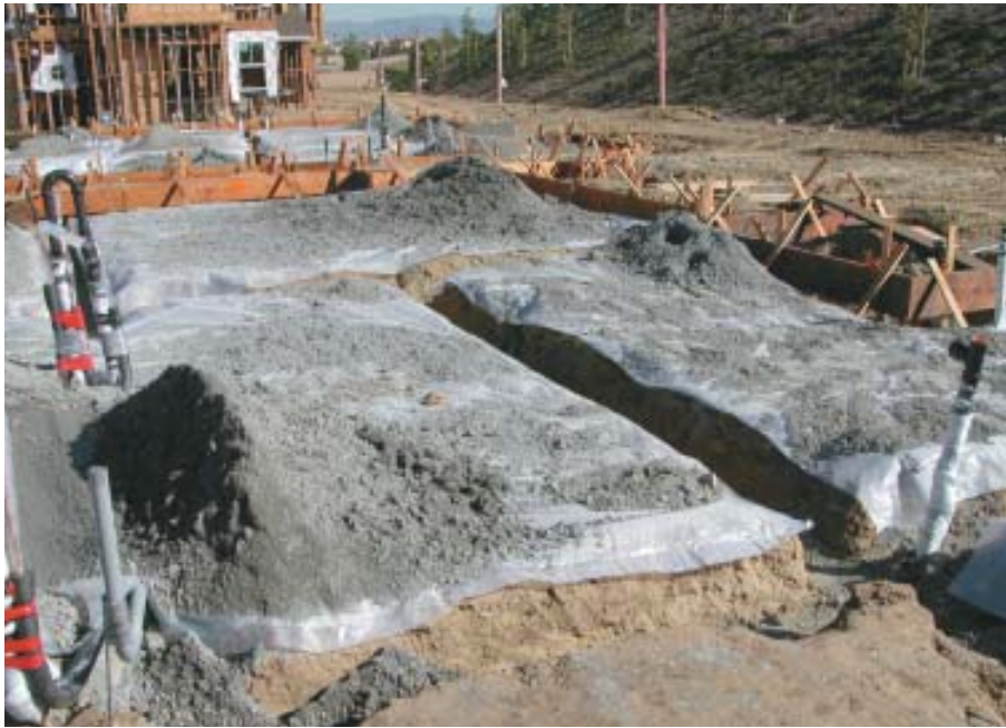
Figure 3. A poly vapor barrier on each soil “block” is held in place with a layer of sand. Where plumbing or conduit runs beneath the bottom of a rib, the excavation is deepened and widened enough to provide the full required thickness and bearing area above and around the buried utility.
