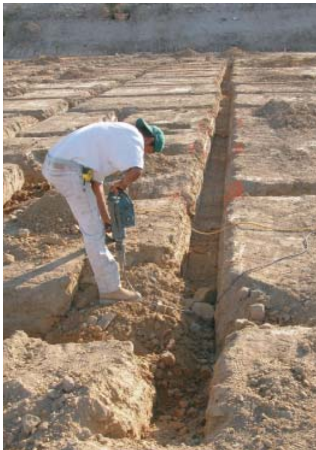
Figure 2. A worker uses a rotary hammer to excavate hard clay that forms the subgrade of a ribbed slab. The network of intersecting trenches defines the internal footings, or ribs, that will stiffen the slab and help it resist soil movement.
